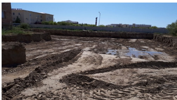
Figure 3 - Place of sampling of soil of the designed building (pit 2.2m deep)
